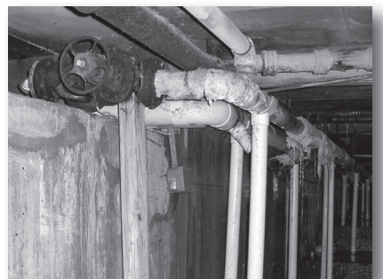
Pool is beyond reasonable repair.
