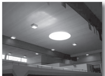
Inadequate lighting and limited natural light.
