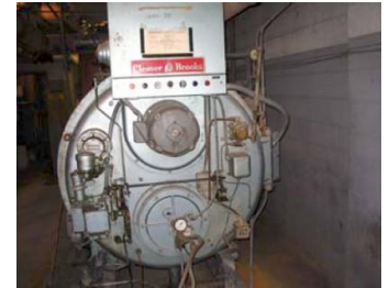
Many building systems have exceeded life expectancy
